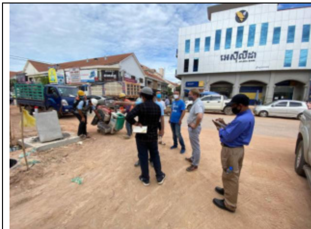
Site visit with Contractor, ongoing works under the "38 roads infrastructure development and rehabilitation"
