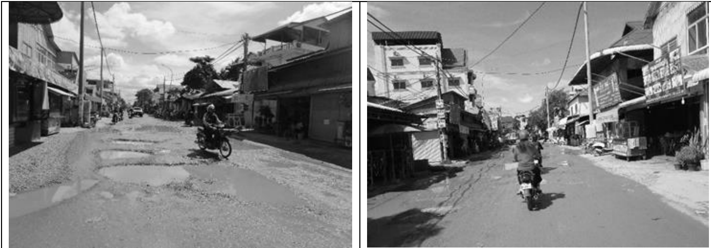
Siem Reap: The poor road section in Vihear Chean village with inadequate side drainage (September 2020)
