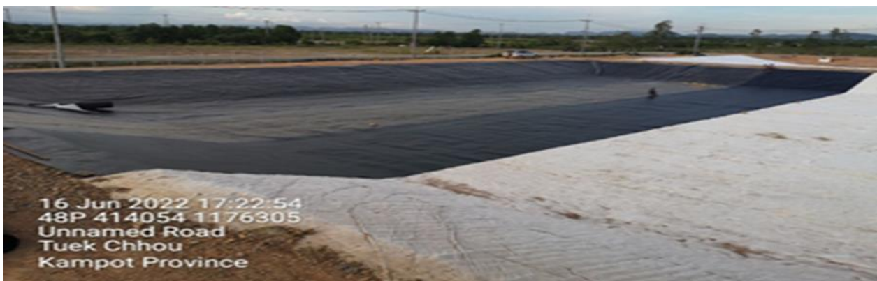
View of Soil filling for embankments and lining at the WWPT site
