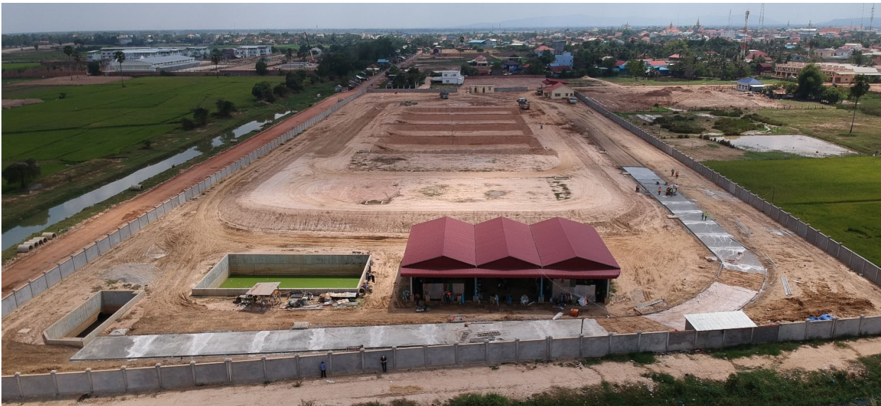
Overview of the Pursat WWTP
