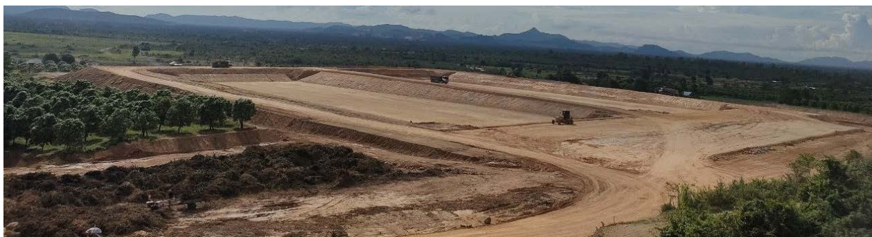
Overview of the landfill construction with earthwork for site development and 2 waste cells completed
