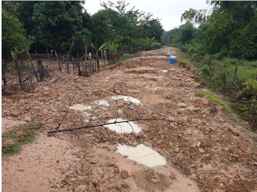
Photo 4-8: Breached section of the river embankment
