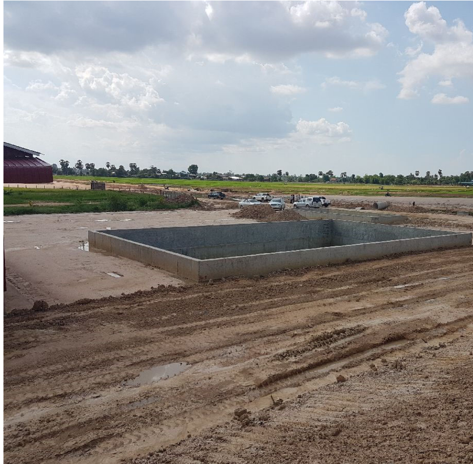
Photo 4-3: Primary settlement and overflow tanks
