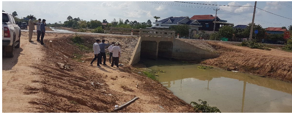
Photo 4-5 Road Culvert in the drainage canal obstructing flow
