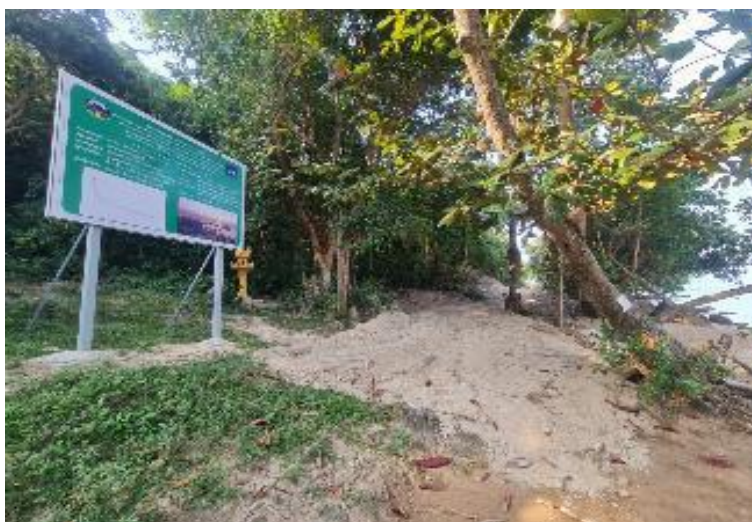
Figure 16. The walkway land clearing and excavation works at PK 0+590 and Project Sign Board
