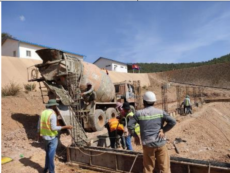
e. Concrete pouring works for the foundation beams of the hazardous cell structure
