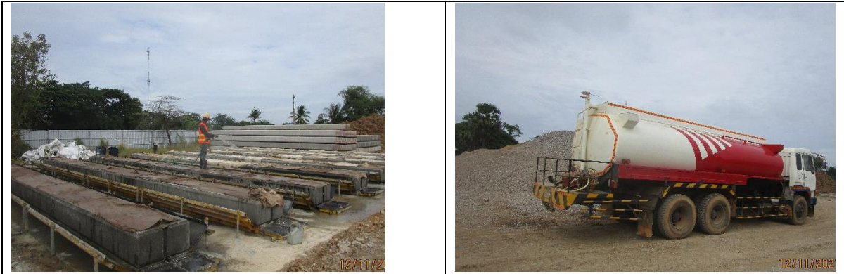
Some construction activities and construction materials and equipment in campsite on November 2021
