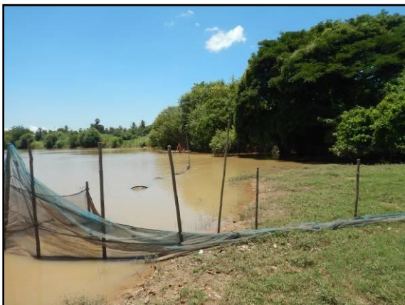
Figure 1-11 River Bank Erosion
